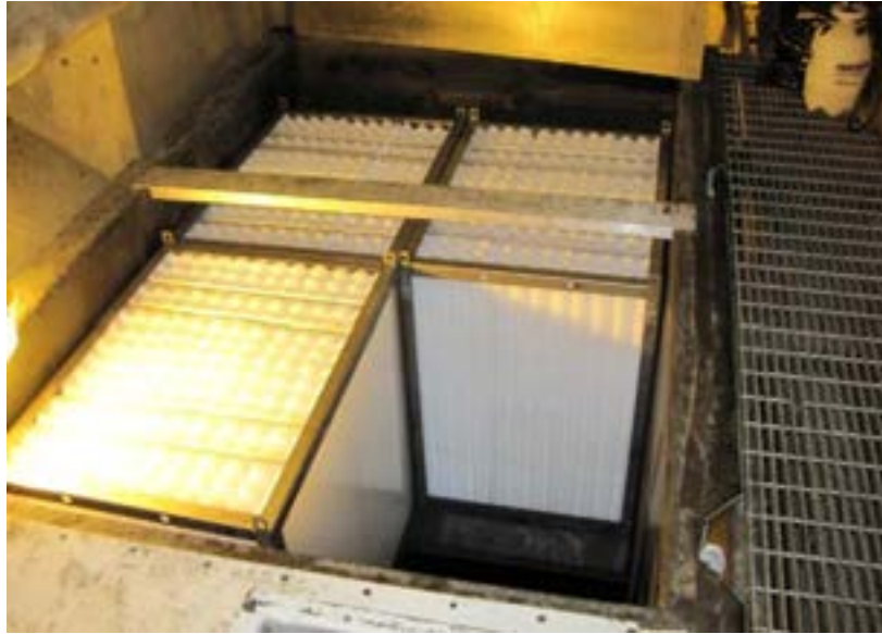
Separator with MSR Media Partially Installed
