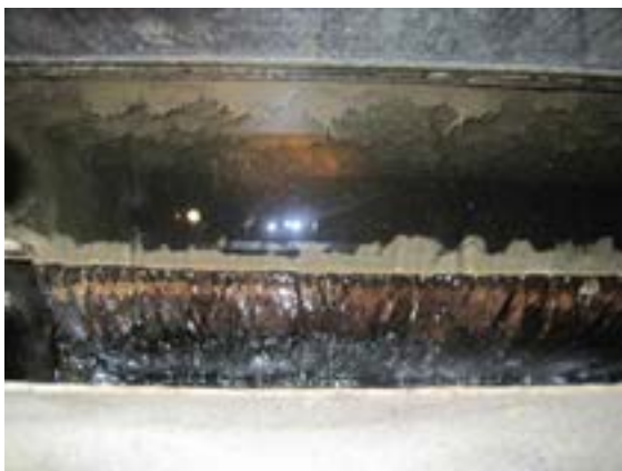
Old Media separator water overflow with substantial bacterial growth
