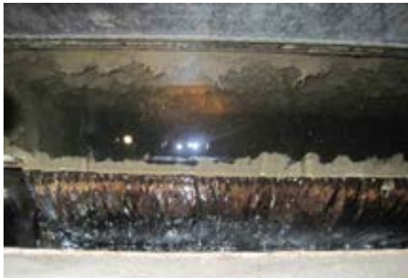
Old Media Separator Water Overflow with Substantial Bacterial Growth
