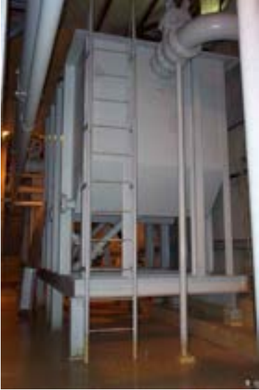
Inlet End View of One Separator
