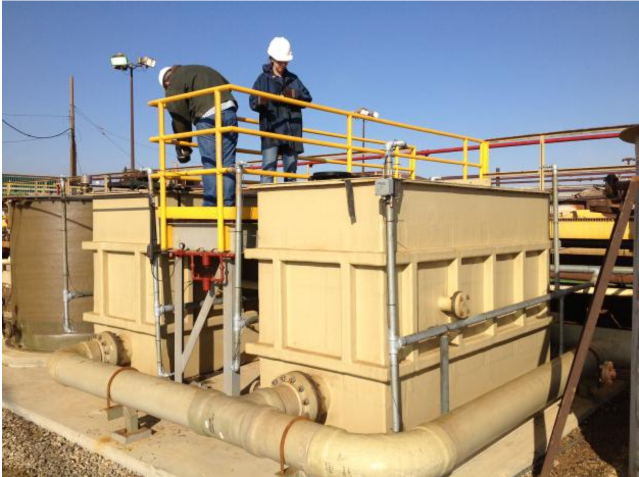
Industrial Brine Processing Separators, two of a set of four
