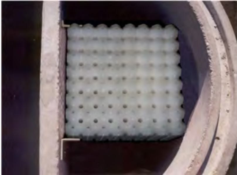
Typical small separator for fuel farm stormwater treatment
