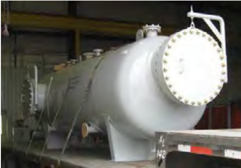
1000 GPM WATER PROCESSING SYSTEM This system is installed at a large natural gas production facility owned by a major oil company.
