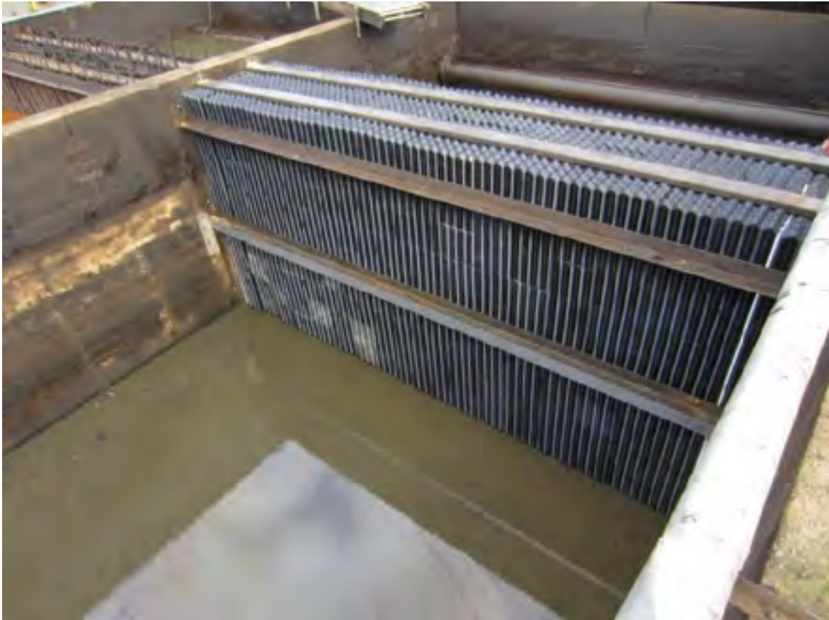
Oil Refinery Effluent Separator: One of a set of four—total capacity 20,000 US gpm (4600 m 3 /hr)
