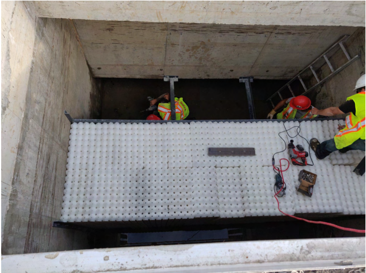
Large Separator at Ottawa, Canada Airport
