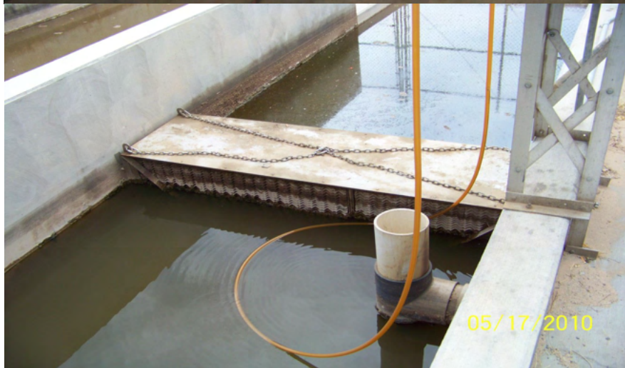
One of nine sys- tems installed in maintenance facilities at 29 palms Marine base in California 2010
